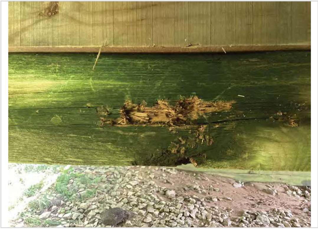
Bent 1 rear side decayed area
